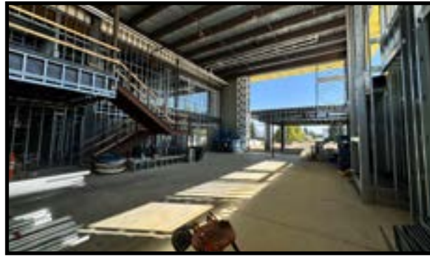
CMMC Cancer Center construction is well underway and on track to open in 2025.
